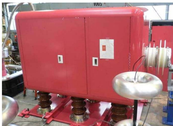
200kV High Voltage Terminal
